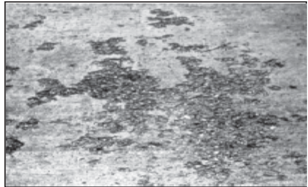
Scaling concrete surface
